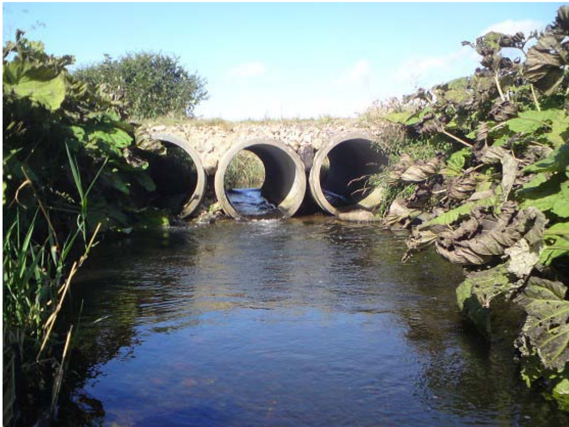
Potential Obstacle, notice perched pipes on either side.
