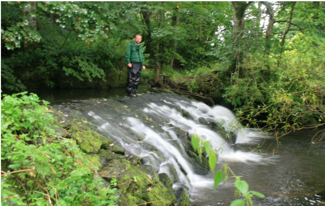
Esset Mill Weir, with Dr Sam Martin standing on structure for scale.
